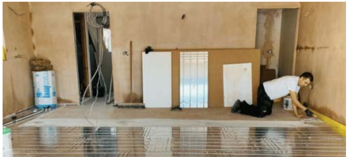
An overfloor system where pipes wrapped in foam sit on top of the subfloor
