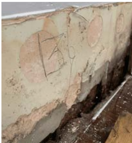
and rising damp was discovered which can be treated
